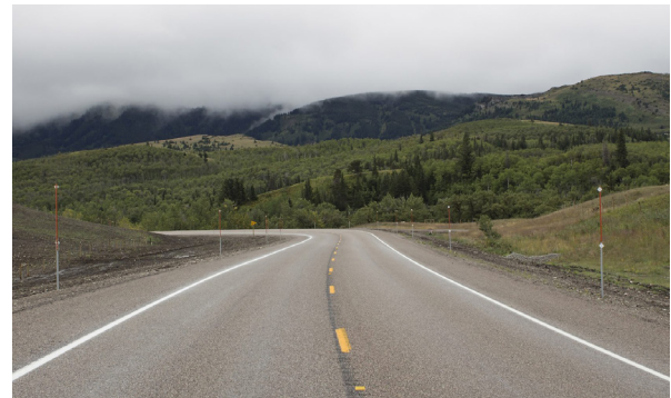
▲ Kiowa Jct N&S and N of Kiowa N | Montana Department of Transportation
