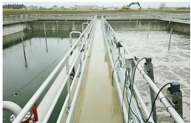
▲ ICEAS Mechanical Wastewater Treatment Plant | City of Glendive
